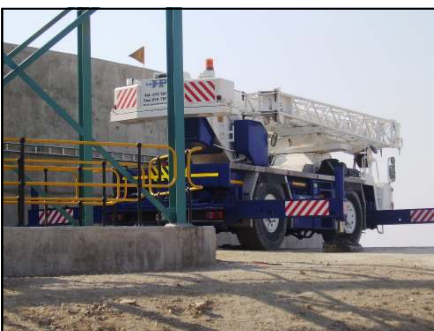
Above: LAC built the crane platforms that are already in regular use.
